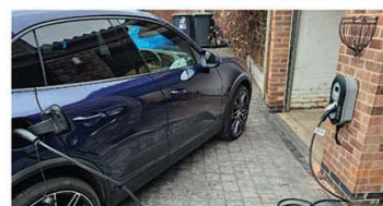
EV CAR CHARGING
